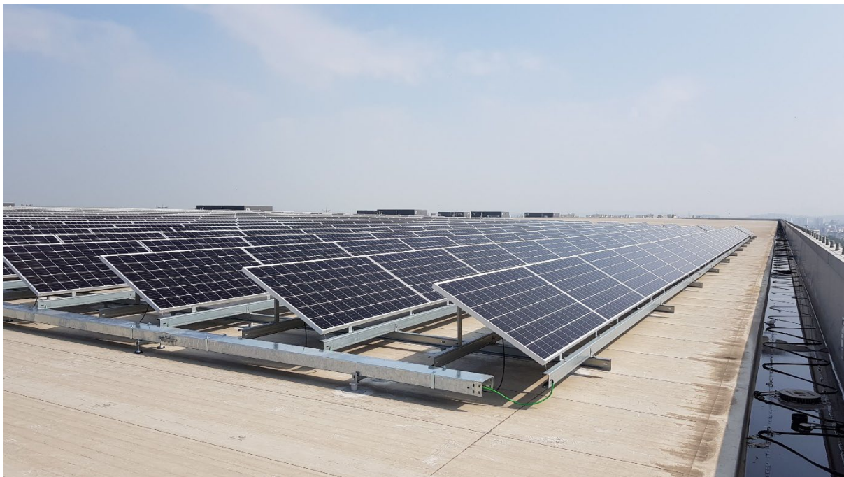
Harnessing solar energy through rooftop solar panels on ESR Group's New Economy assets in South Korea
